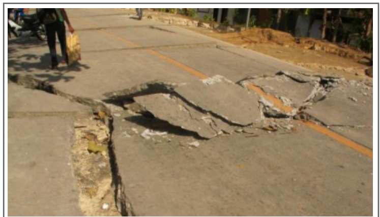
SHIFTED PAVEMENT ON A HIGHWAY AFTER A 7.2 MAGNITUDE QUAKE HIT THE CENTRAL PHILIPPINE ISLAND OF BOHOL ON OCTOBER 15 WITH A DEATH TOLL OF 222. [PHOTO BY MOISES MUSICO, ADRA-PHILIPPINES]
